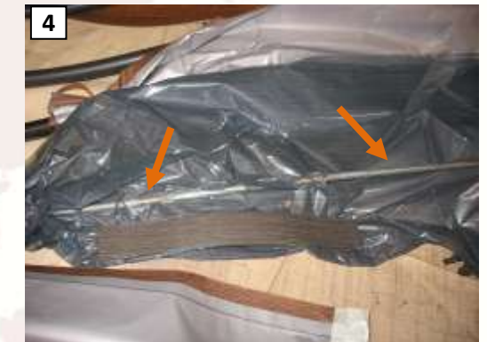
4 It is important to let the film perfectly adhere on the whole surface to decorate: this is why an additional suction pipe may be used inside of the bag (orange arrows)
